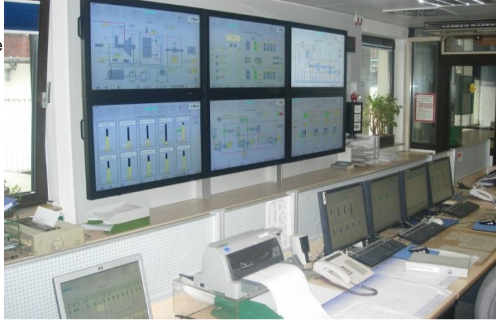
Switch room power station machine house 2
