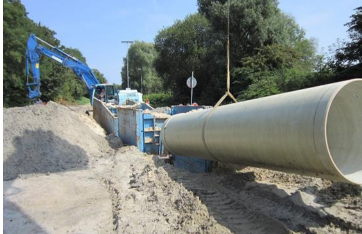
Pressure sewer DN 1200 at the Pumping Station South
