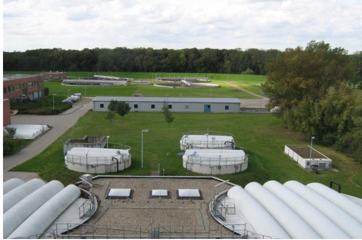
Waste water treatment plant of Dessau-Rosslau
